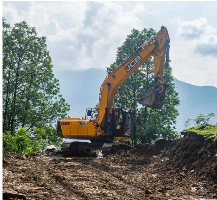
An excavator digs into the topsoil surrounding Ghandruk to build a road connecting it to the nearby village of Little Paradise. As primitive as it looks, this road is considered finished.
